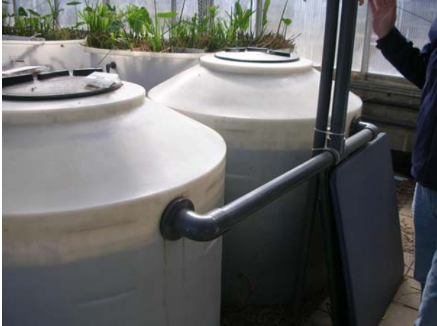
Aerobic Tank Vents
